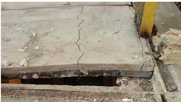
(b) R-C slab edge transverse cracking
