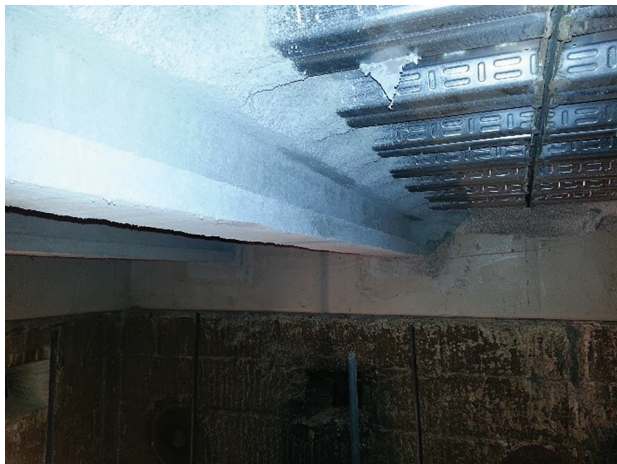
(a) Typical SFRM-protected beam (showing the longitudinal seam between slabs of adjacent specimens)
