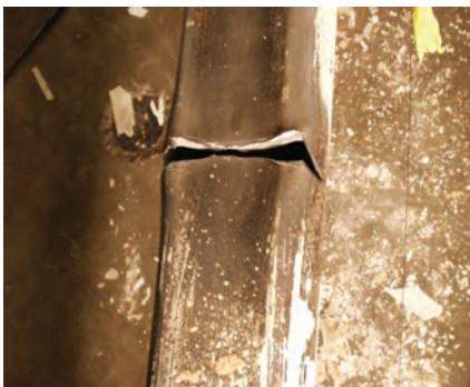
(e) Ductile tearing initiates at corners and progresses across the tube wall
