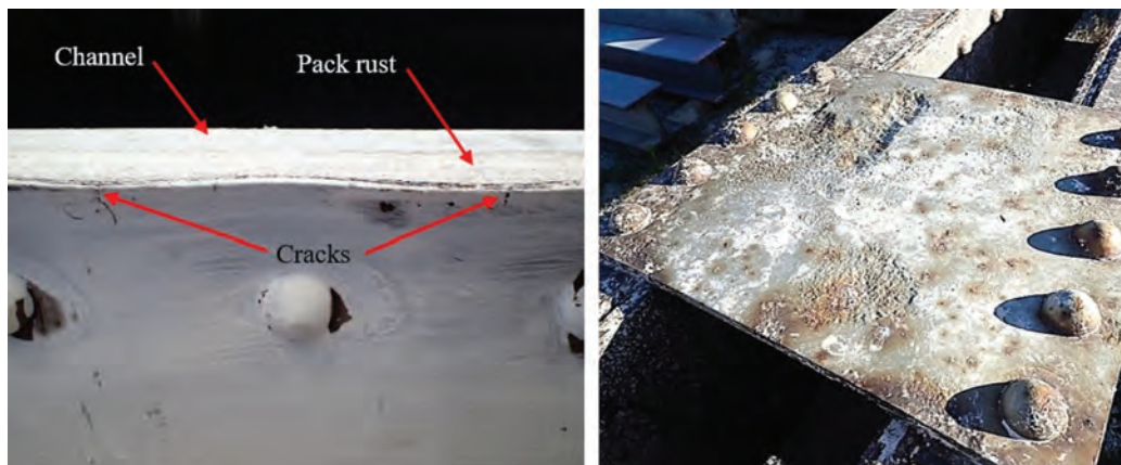
Fig. 3. (Left) Specimen 2 (whitewashed for testing) showing defects and section loss; (right) typical section loss of a stay plate.
