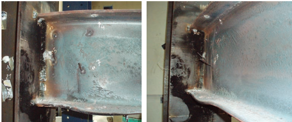
Fig. 21. Local buckling on the beam bottom flange and shear buckling of the beam web (joint Z2).
