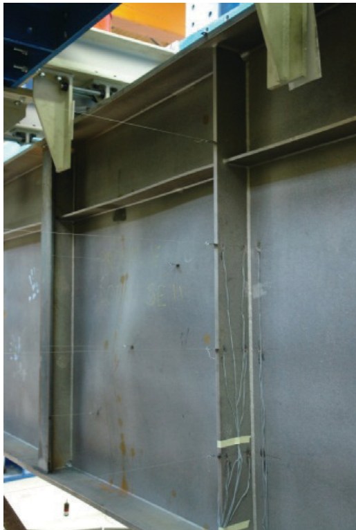
Fig. 7. Plate girder test to assess the influence of tension field action on the transverse stiffener. (Photograph courtesy of Professor Darko Beg)
