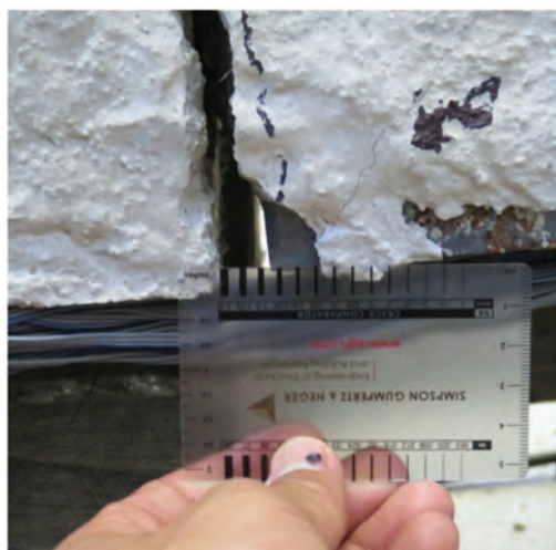
(a) Gap opening at the RC-SC interface
