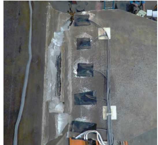
(b) Top-flange fracture
