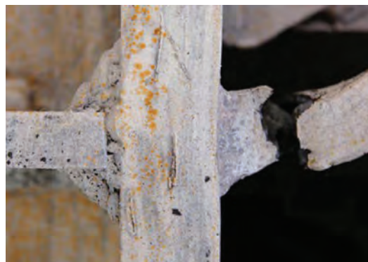
(b) Fracture 2 at bottom flange
