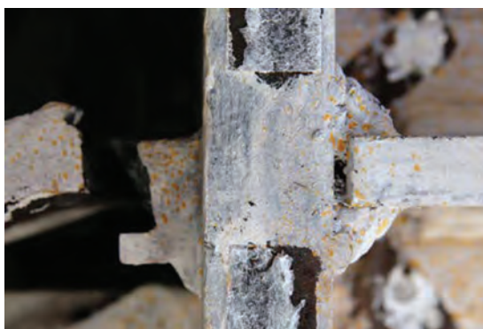
(a) Fracture 1 at top flange
