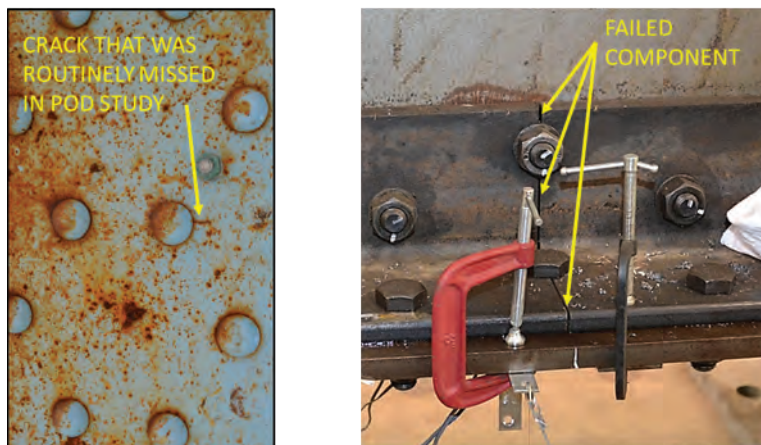
Fig. 1. Photographs of two different cracks in built-up members contrasting the differences in cracks that need to be detected in a traditional FCM inspection vs. those associated with an IRM.
