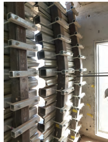
(b) HSS members after field test, with displacement transducers, illustrating global failure of members due to far-field air-blast
