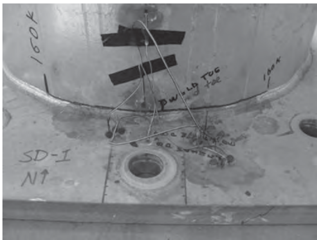
Fig. 11. Cracking on south face of AB_1.
