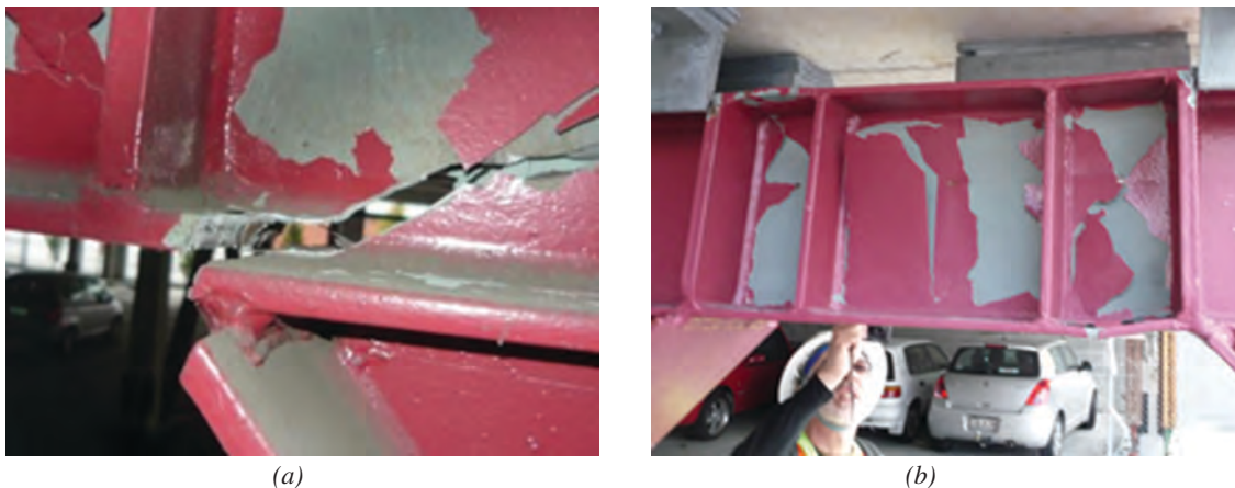
Fig. 1. Photos of EBFs taken inside a parking garage following the Christchurch earthquake of 2011 (Clifton et al., 2011): (a) fractured EBF (lower level); (b) evidence of plastic action without fracture (top level).
