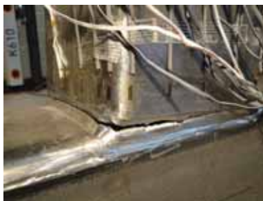
(k) T-1.00-23: weld rupture
