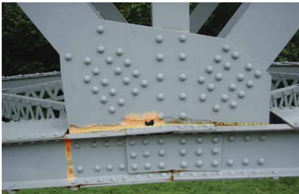
Fig. 6. Narrow band of section loss in gusset plate just above chord member.
