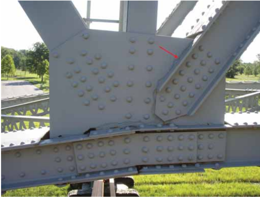
Fig. 10. Pitting a long top flange of diagonal member (WMN pitting).
