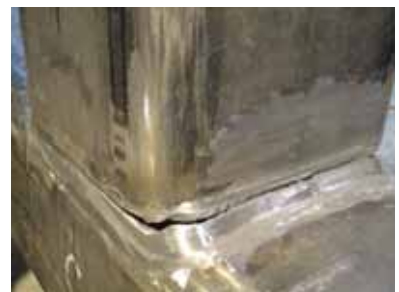
(l) T-1.00-17: weld rupture
