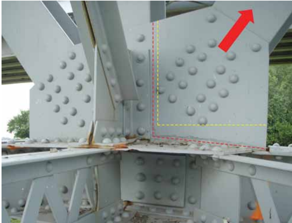
Fig. 7. Gusset plate corner resisting tension generated by diagonal web member.
