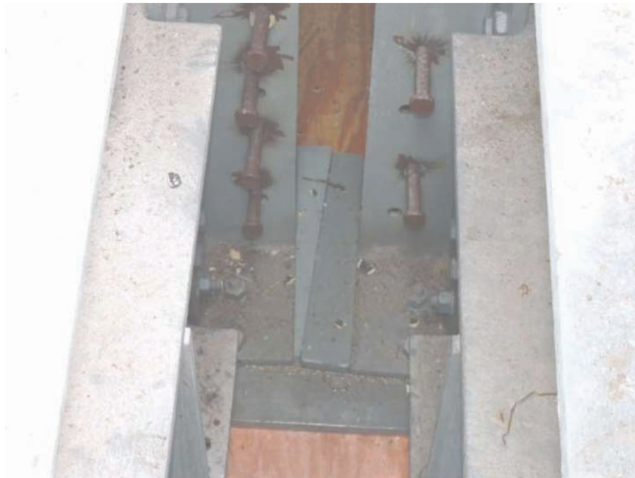
Fig. 4. Wedge plates between bottom flanges of adjacent-span stringers (Section RES construction photo).
