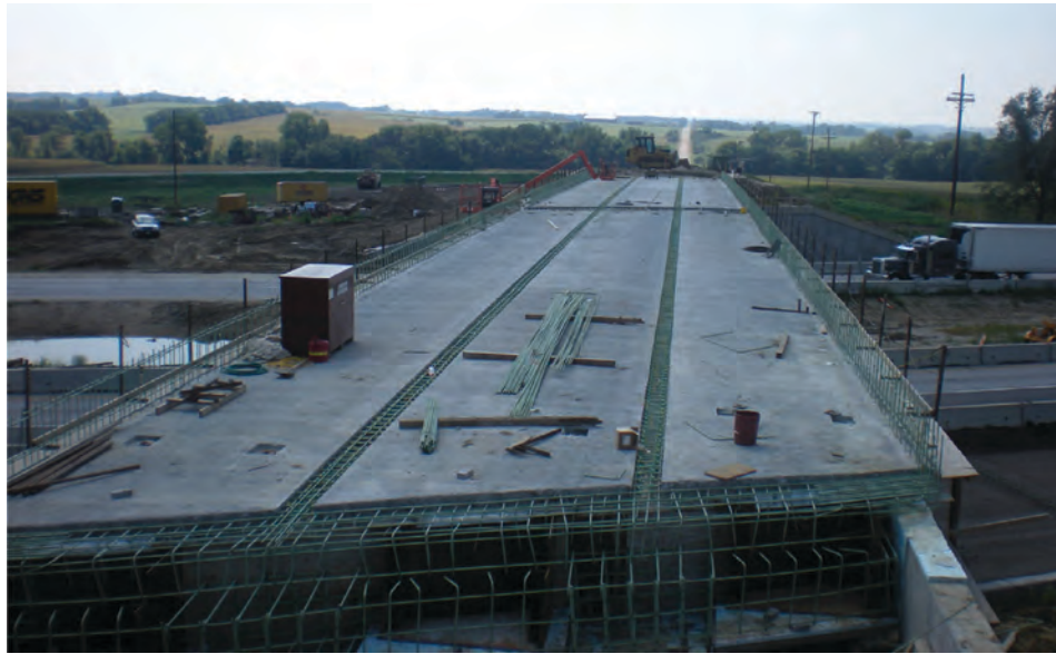
Fig. 18. Completing the placement of the pre-topped units for the bridge over I-80 at 262nd Street in Nebraska.
