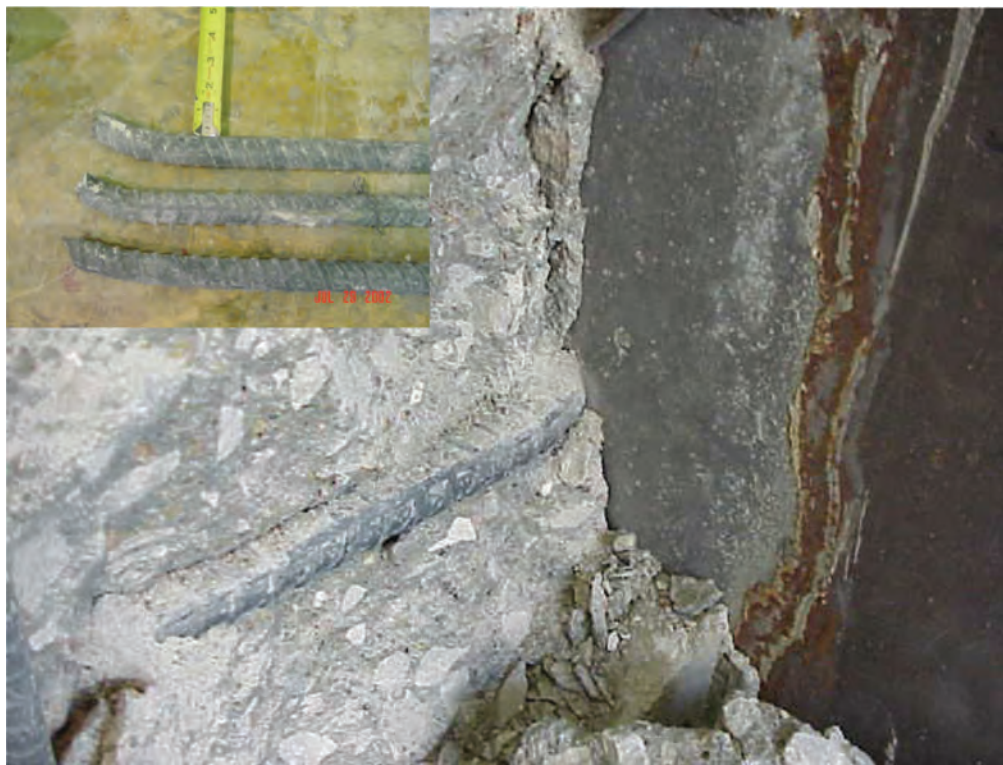
Fig. 23. Shear failure of the transverse bar inside the diaphragm after the conclusion of the ultimate test—specimen 2.
