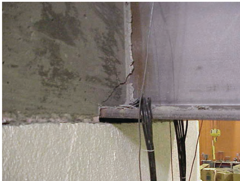
Fig. 22. Cracking of the concrete diaphragm around the bottom flange—specimen 2.
