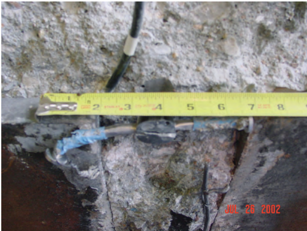
Fig. 18. Gap between bottom flanges.
