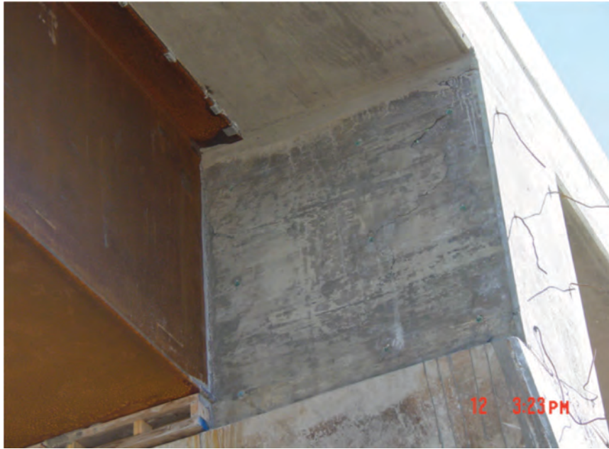
Fig. 12. An example of cracking in the concrete diaphragm if it is cast full depth.
