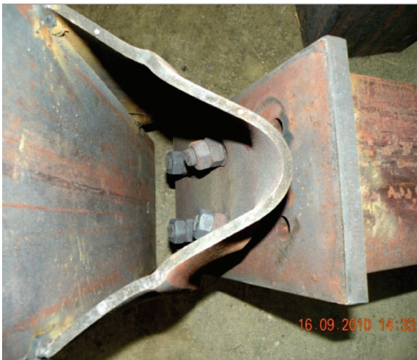
Fig. 3. Typical failure mode of a reverse-channel connection (photograph courtesy of Professor Ian Burgess).
