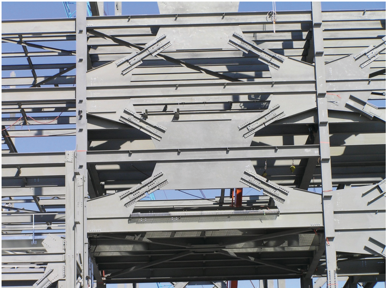
Fig. 4. An example of the barn-door gusset effect.
