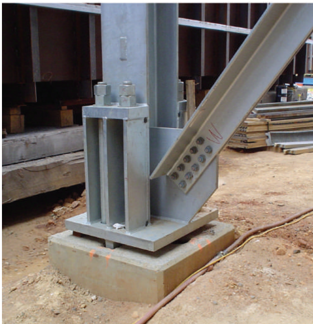
(a) Base chair for heavy industrial facility
