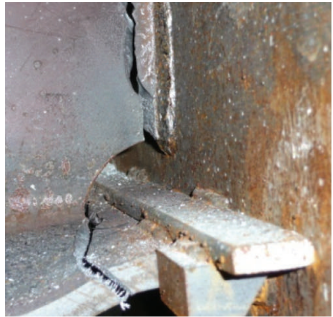
Fig. 2. Failure mode of older beam-to-column connection. (Photo courtesy of Professor M. Nakashima)
