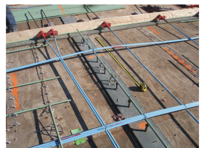
(c) Beam B at girder 2.
