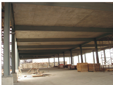
(f) Completed structure looking North; beams B, C and D in far background.
