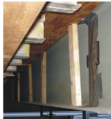
(c) Gauge installation showing form shore installed on top of gauge at this location.
