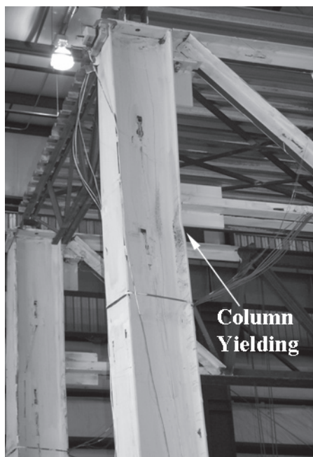
Fig. 11. Plastic hinge formation at the column.
