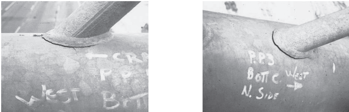
Fig. 12. Typical cracking observed during sign support structure service life.
