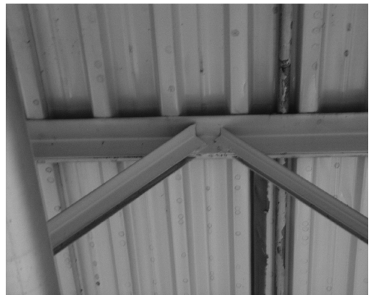
Fig. 5. Angles interfering with top chord reinforcement.
