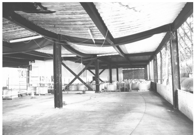
Fig. 1. Deflected shape of the Cardington frame after the “BS Corner Test.”
