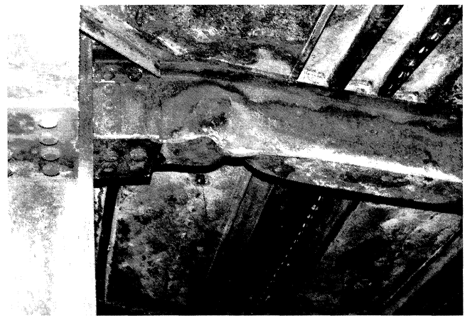
Fig. 8. Severe local buckle in beam.
