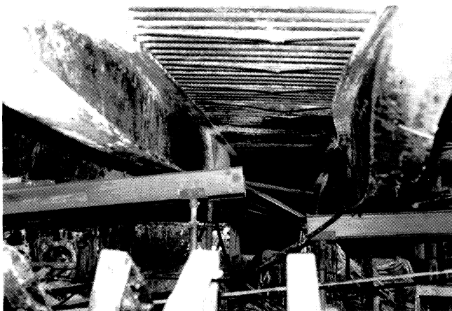
Fig. 7. Considerable thermally induced beam twisting.
