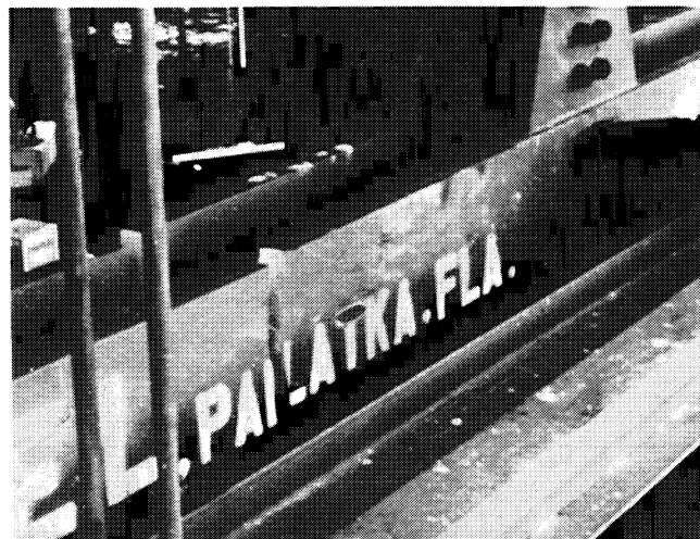
Fig. 1. Fractured chord of Orlando Civic Center truss
