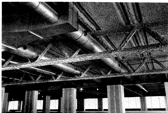
Fig. 4. Passage of mechanical ducts through truss
