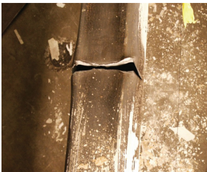
(e) Ductile tearing initiates at corners and progresses across the tube wall
