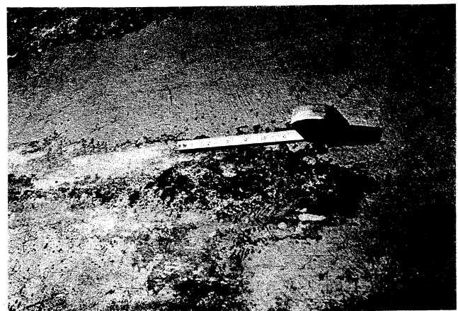
Fig. 6. Deeper corrosion pits, observed infrequently. Surrounding area unaffected by corrosion. Typical profile in Fig. 7c
