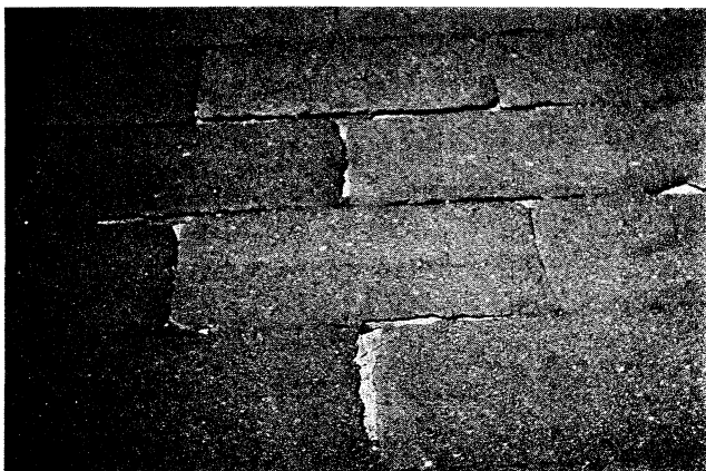
Fig. 2. Deteriorated original planking, Bronx-Kill Bridge
