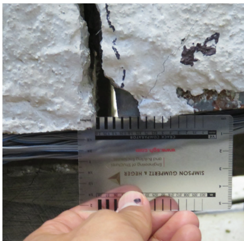
(a) Gap opening at the RC-SC interface
