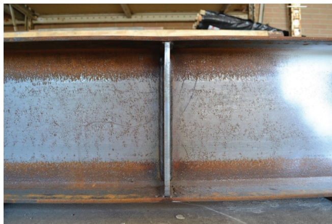
Fig. 13. Elevation view of W12×26 DC-E0 after testing.
