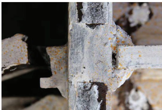
(a) Fracture 1 at top flange
