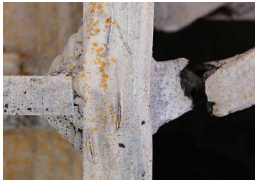
(b) Fracture 2 at bottom flange
