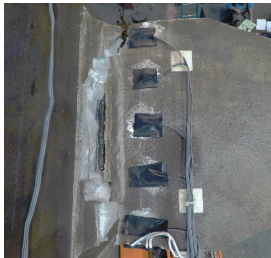
(b) Top-flange fracture
