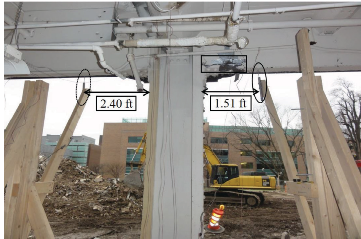
Fig. 6. Vertical LVDT to the south (in circle on left) and north (in circle on right) of the removed column and horizontal LVDT (rectangle) attached to the removed column.
