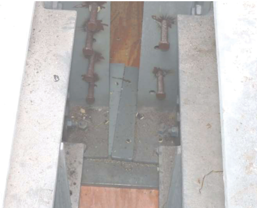
Fig. 4. Wedge plates between bottom flanges of adjacent-span stringers (Section RES construction photo).
