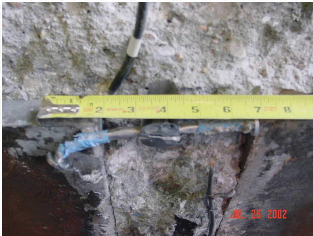
Fig. 18. Gap between bottom flanges.
