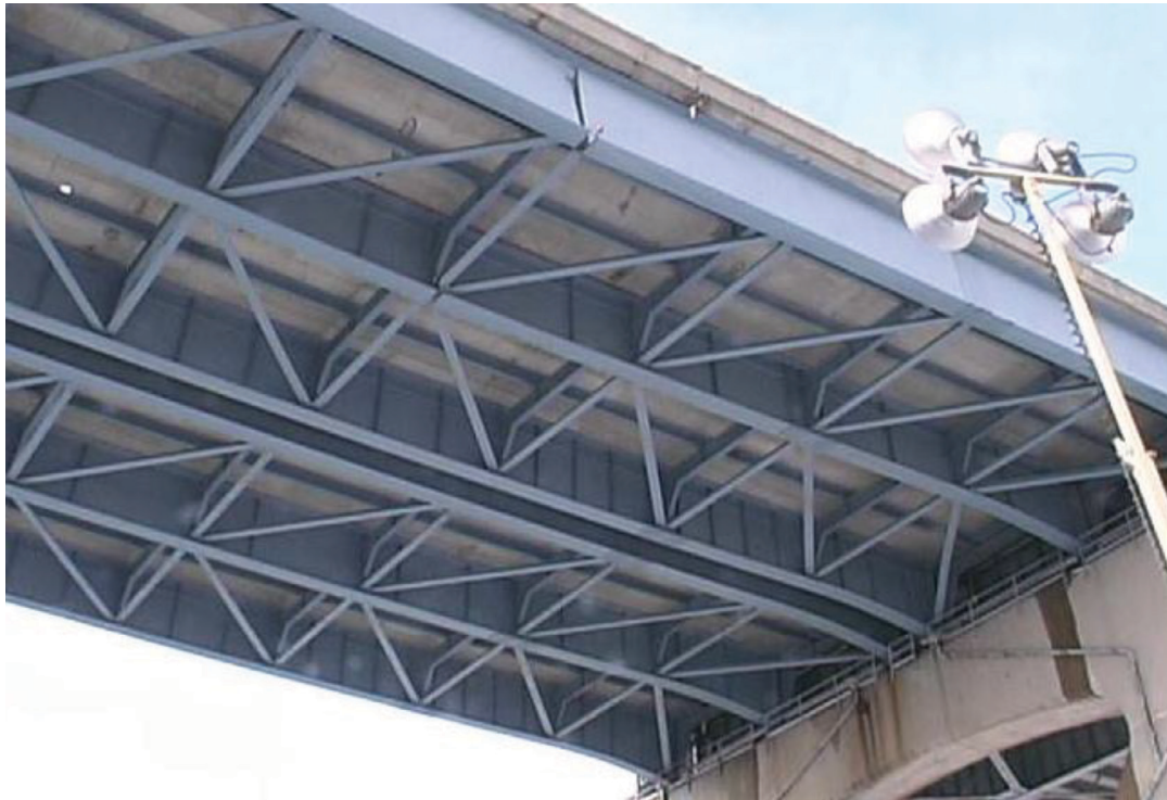
Fig. 11. Two of three girders with full-depth fractures in the Hoan Bridge in Milwaukee, Wisconsin (photograph courtesy of Professor William Wright).
